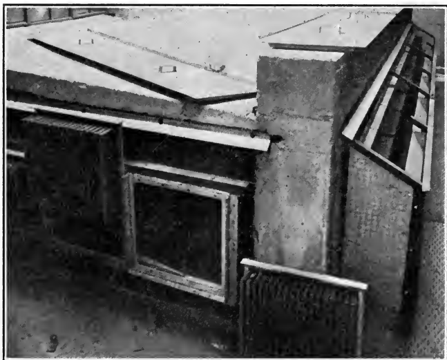
FIG. 6. Felt filters installed at West Coast studio.
